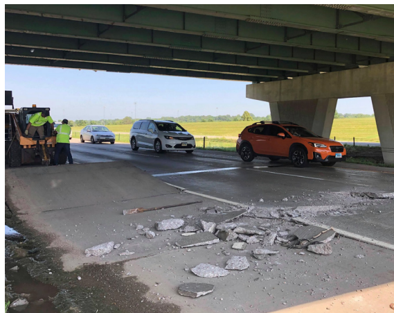
Roads buckling in extreme heat
