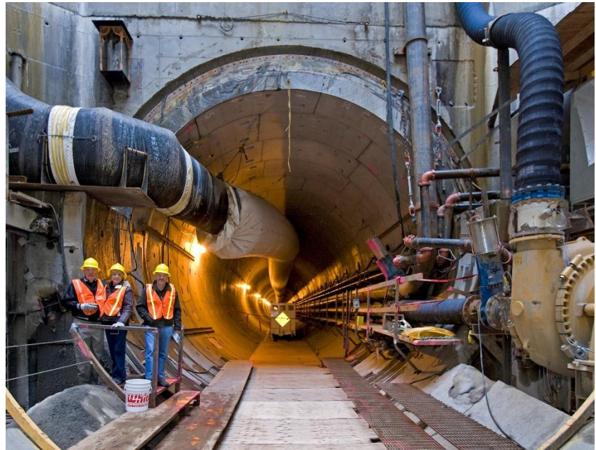
An inside view of Portland's Big Pipe's east side tunnel. This section of tunnel is known as Opera Shaft, as the tunnel sits below the property of the Hampton Opera Center.
