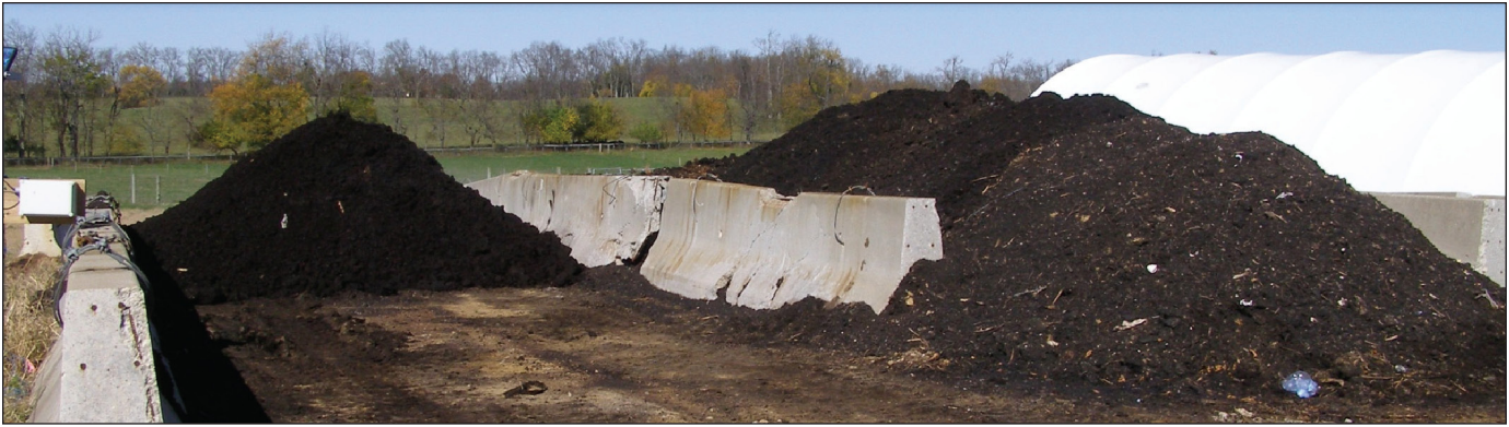
Figure 4. Example of a bin composting system constructed using soil cement flooring and construction barriers.
