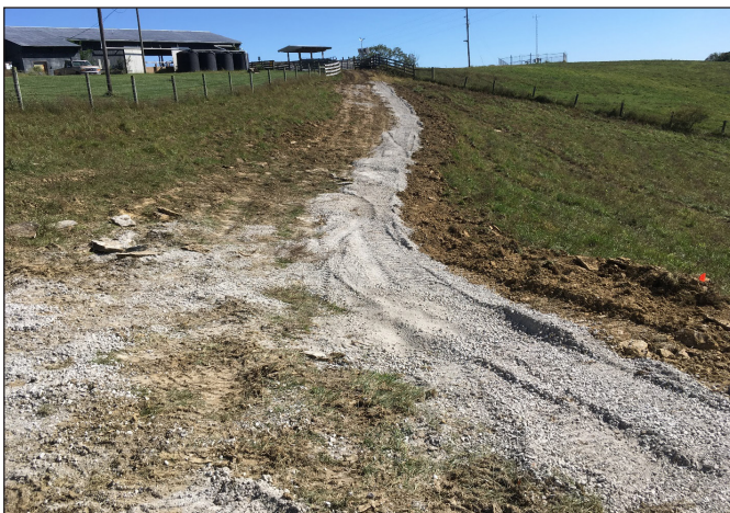
Figure 6. A completed trail leads to a water source located on a hill with 30-percent slopes.
